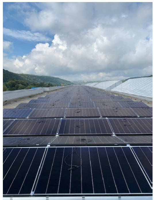
Photovoltaic system at the Dörzbach site
