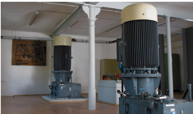
Hydro-electric power station on the river Kocher
